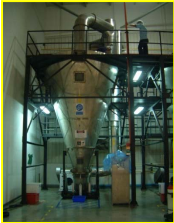
Supply and Install Cyclone Dryers Cardinal Health– 3 sets, Project Value:- 9 million baht
