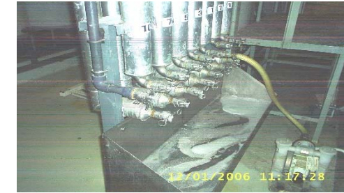
Premixing tank @ Chlorination
