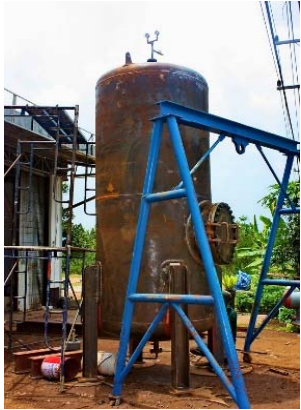
Air Receiver Tank Client: Cardinal Health Location:- Amata City Compny:- USA
