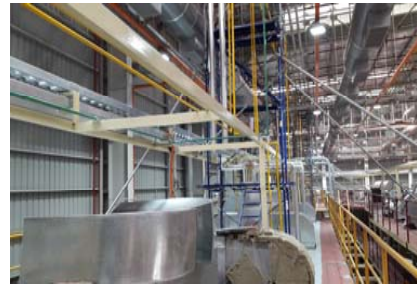
Exhaust Duct@ Pineapple project
