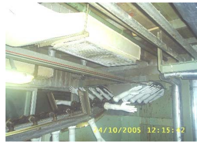
Aurcon Duct @Stripping Station
