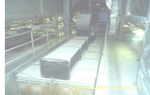
AHU @ Line J and Line K
